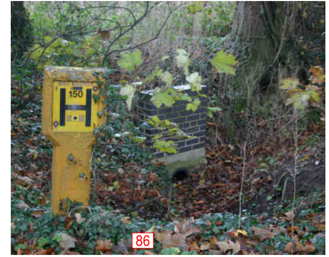
Fig 28 Hydrant at the ditch near White Mill [86]
