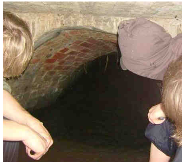
Fig 17 Brick-lined culvert under the mini-roundabout, thought to be looking N along Grape Lane
