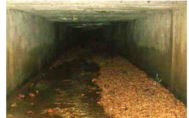
Fig 18 Concrete culvert under the mini-roundabout, thought to be looking NE along Railway St.
